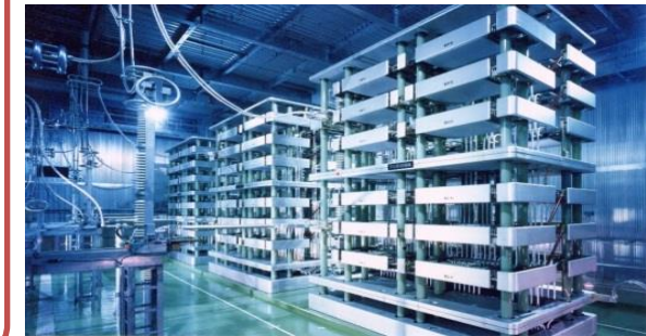
Kii Channel HVDC converter
